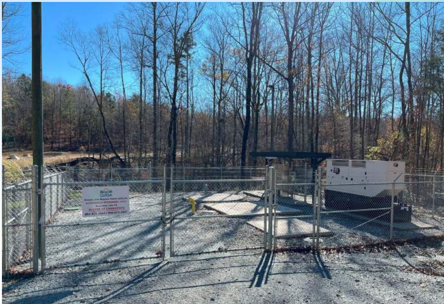
I-85 Sewer Phase II: Broomway Lane Pump Station
